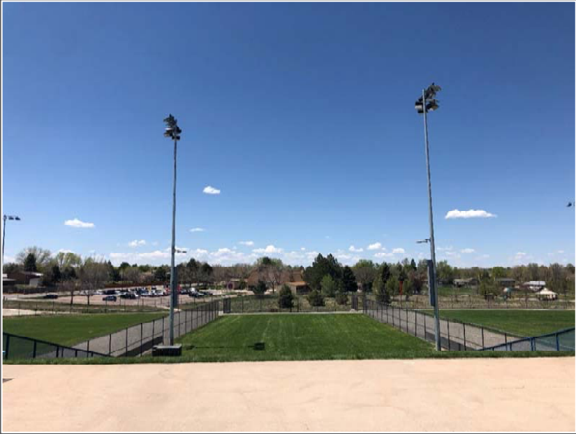
New LED Lights
