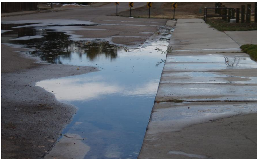
SEVERE SUNKEN "BIRD-BATH"
